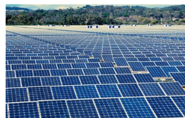
A solar farm.
